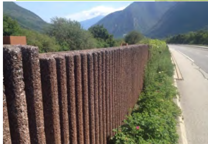
Highway acoustic panel barriers
